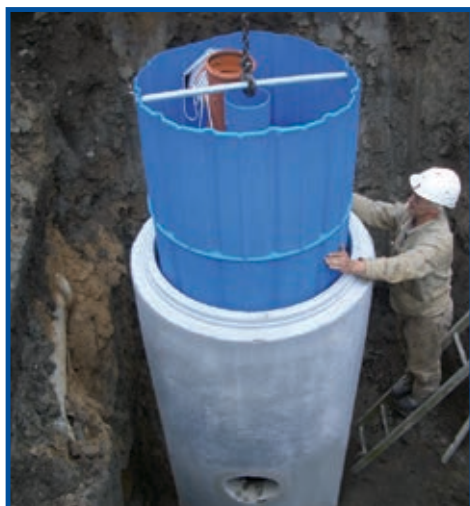
Hydrofilter 1000 monteras i befintlig 1000 brunn.
